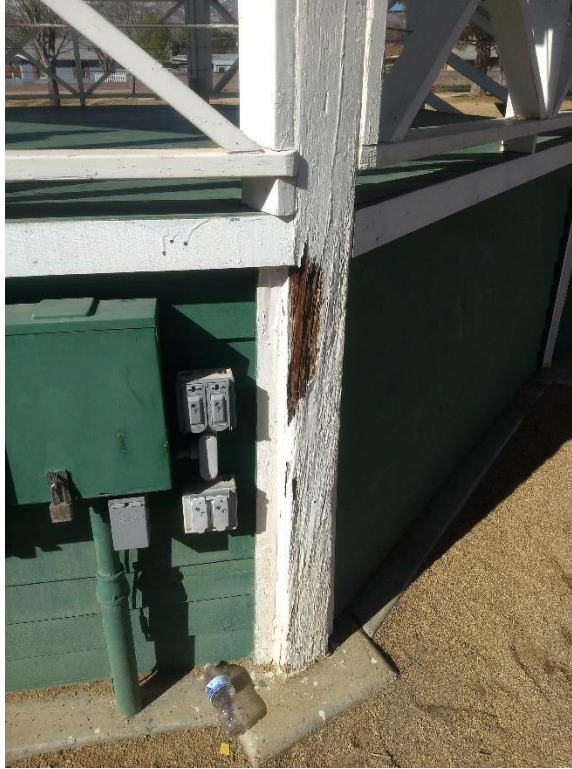
Figure 7: 6x6 post deteriorating near floor level.
