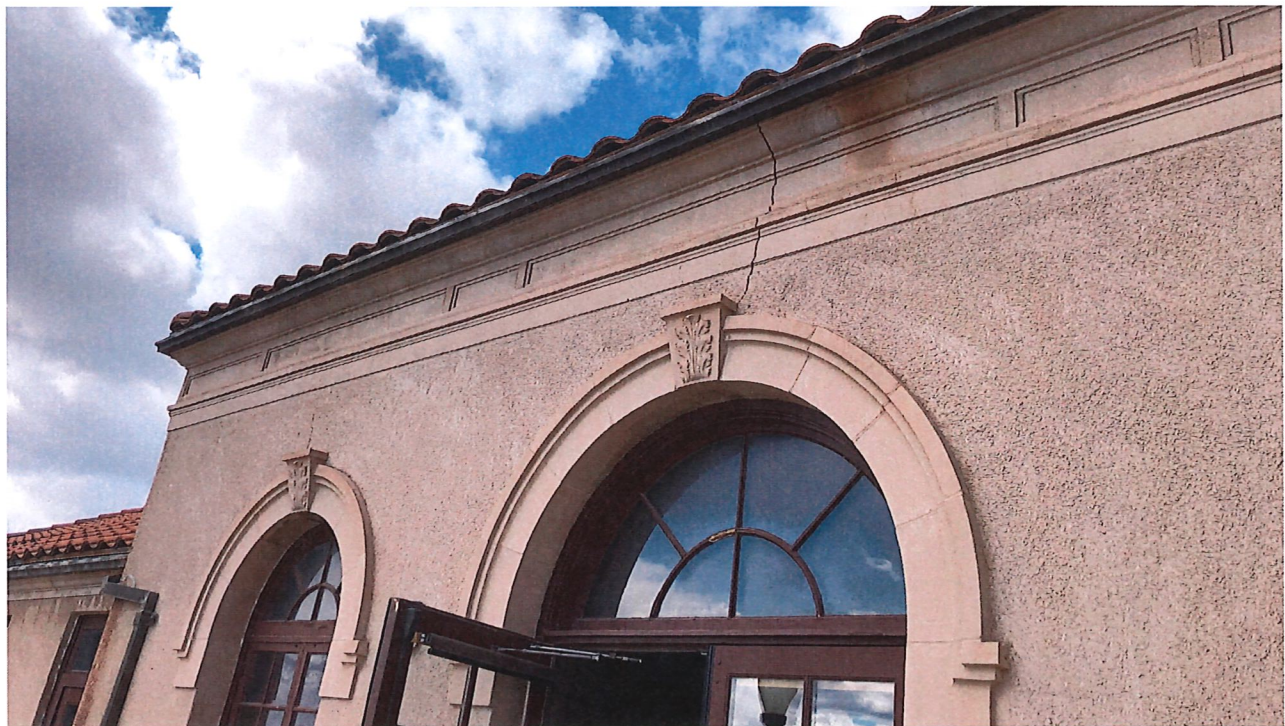
Photo 4 – Crack over Doorway of Clubhouse
