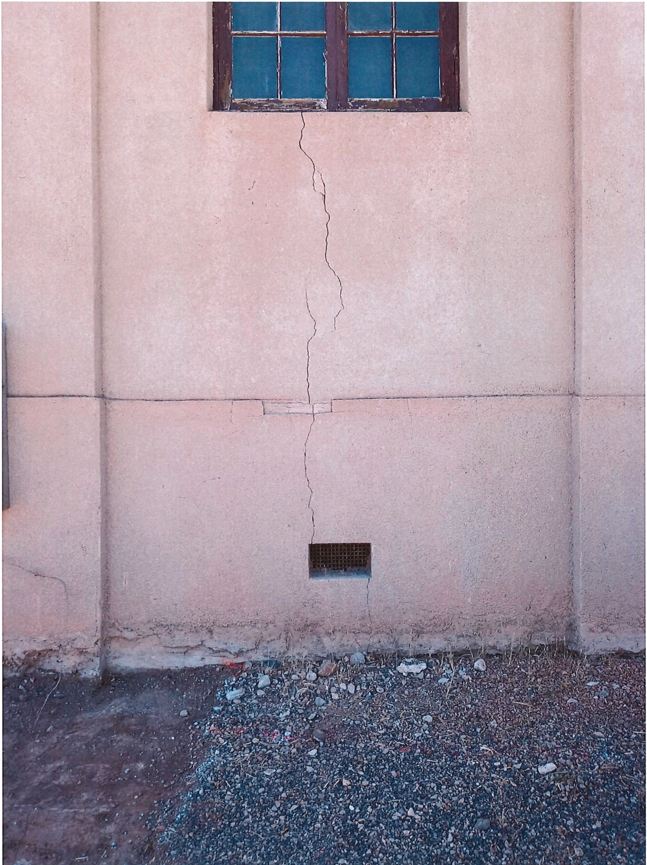
Photo 8 – Cracks in Wall
