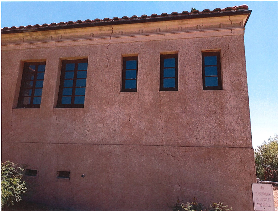
Photo 10 – Multiple Cracks in Wall, Memorial Building, South End, West Side
