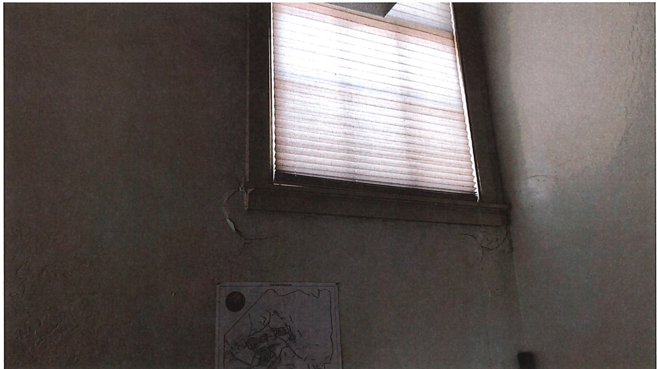
Photo 2: Window Damage - Public Works Building
