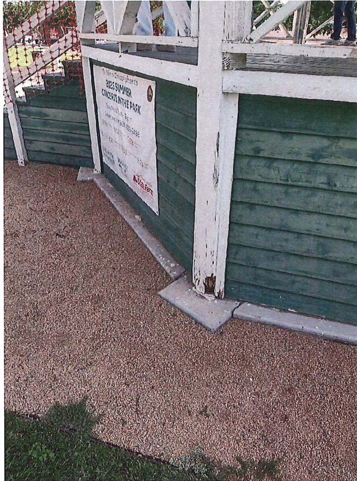
Photo 8 – Poor condition at base of column
