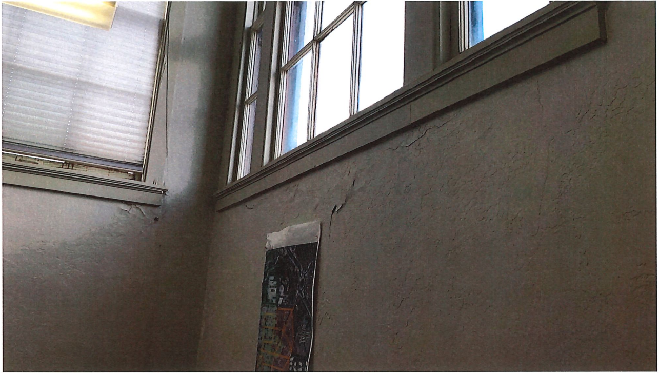
Photo 3: Window Damage - Public Works Building
