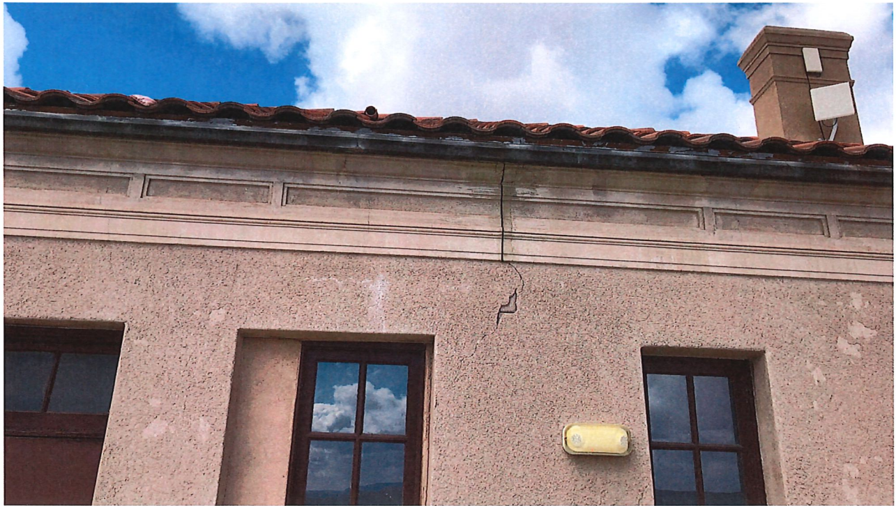
Photo 5 – Large Crack at soffit and below, Memorial Building
