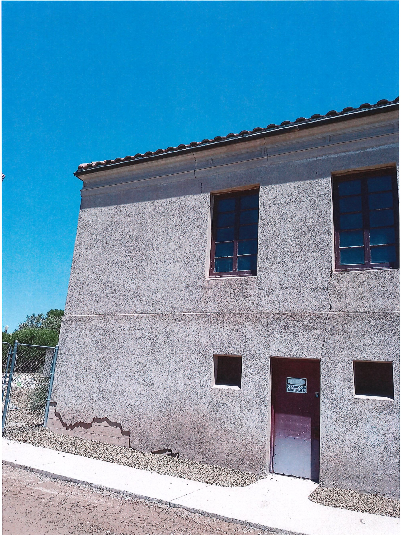
Photo 11 – Stucco Loss, Memorial Building, South Side
