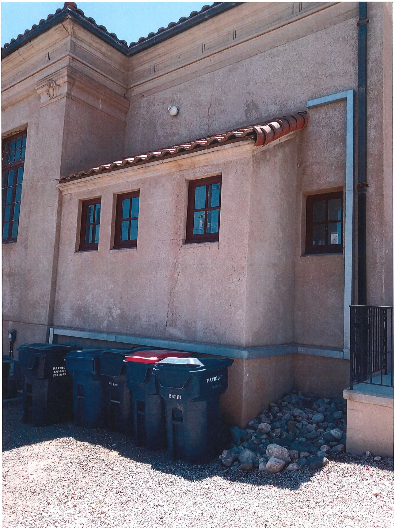
Photo 7 – Cracks in Wall, Memorial Building, North Side
