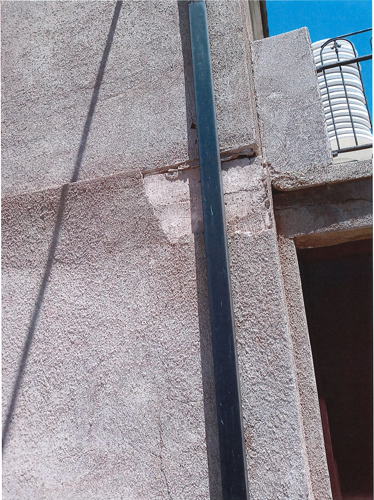
Photo 9 – Cracks at Doorway, Memorial Building, South Side
