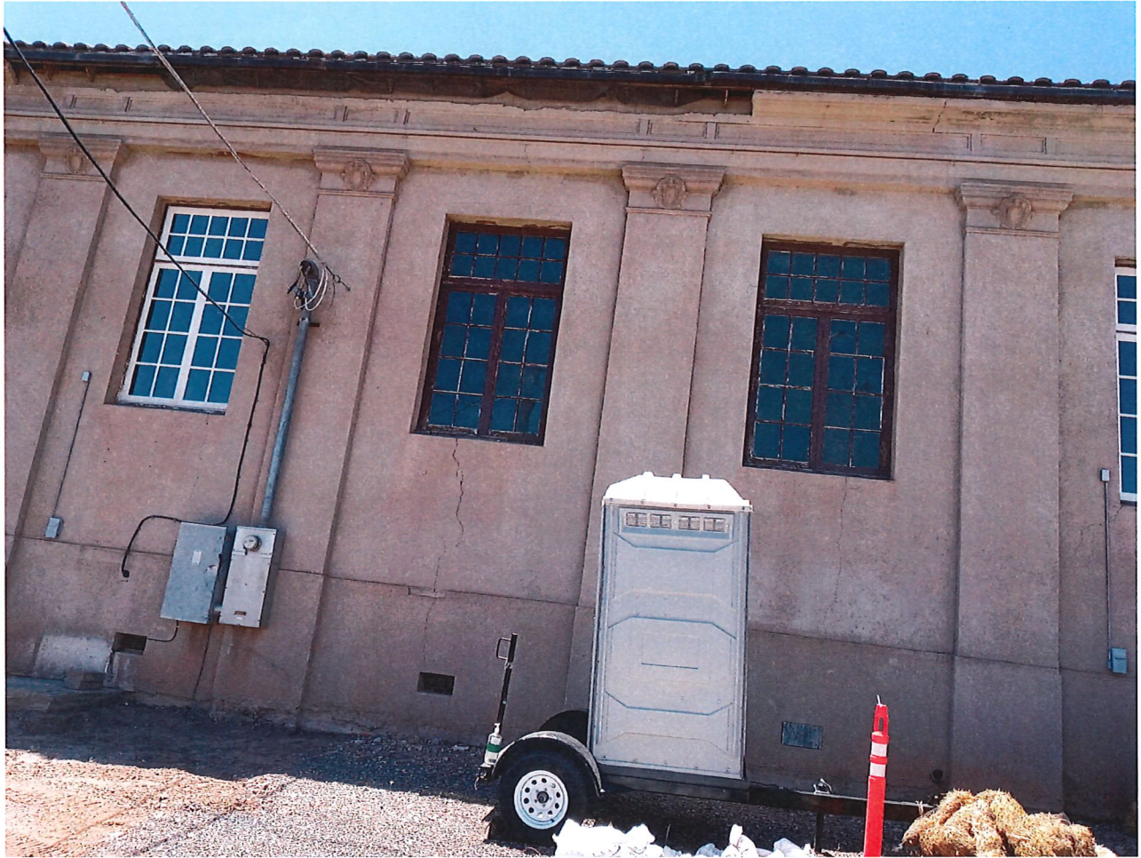
Photo 12 – Soffit missing - Memorial Building – North Side
