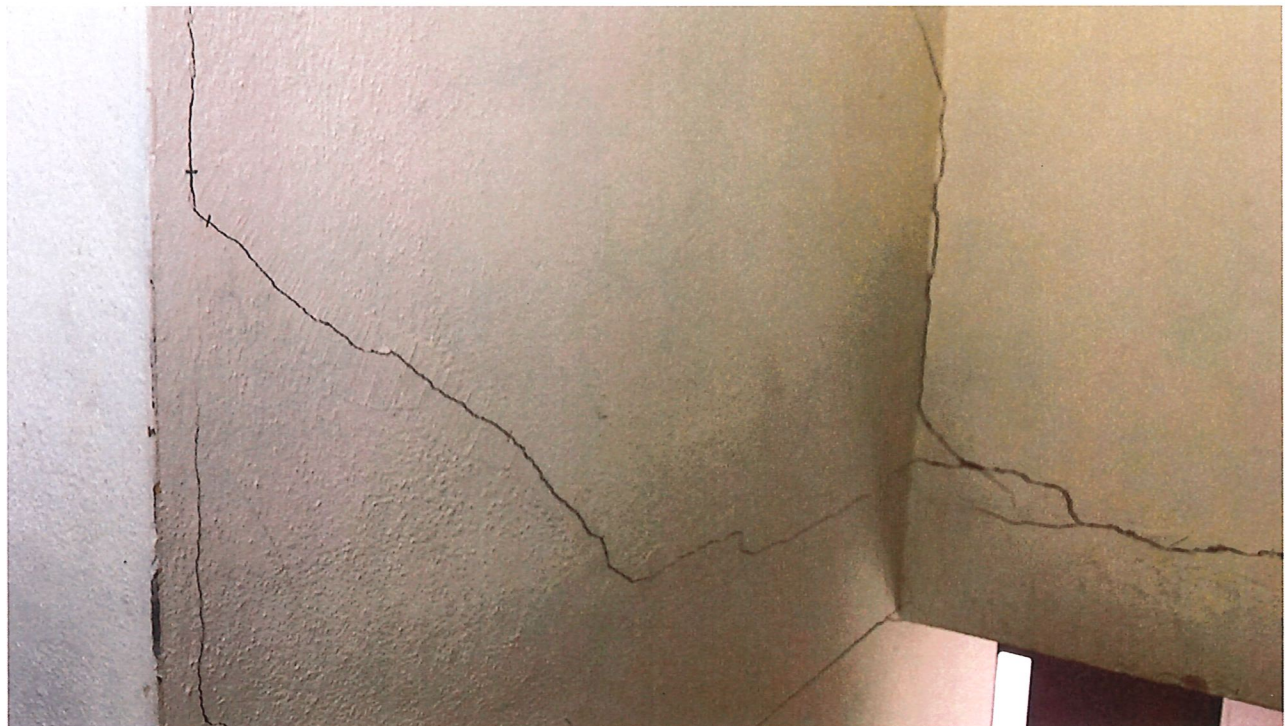
Photo 13 – Wall Crack at Stairwell of Library
