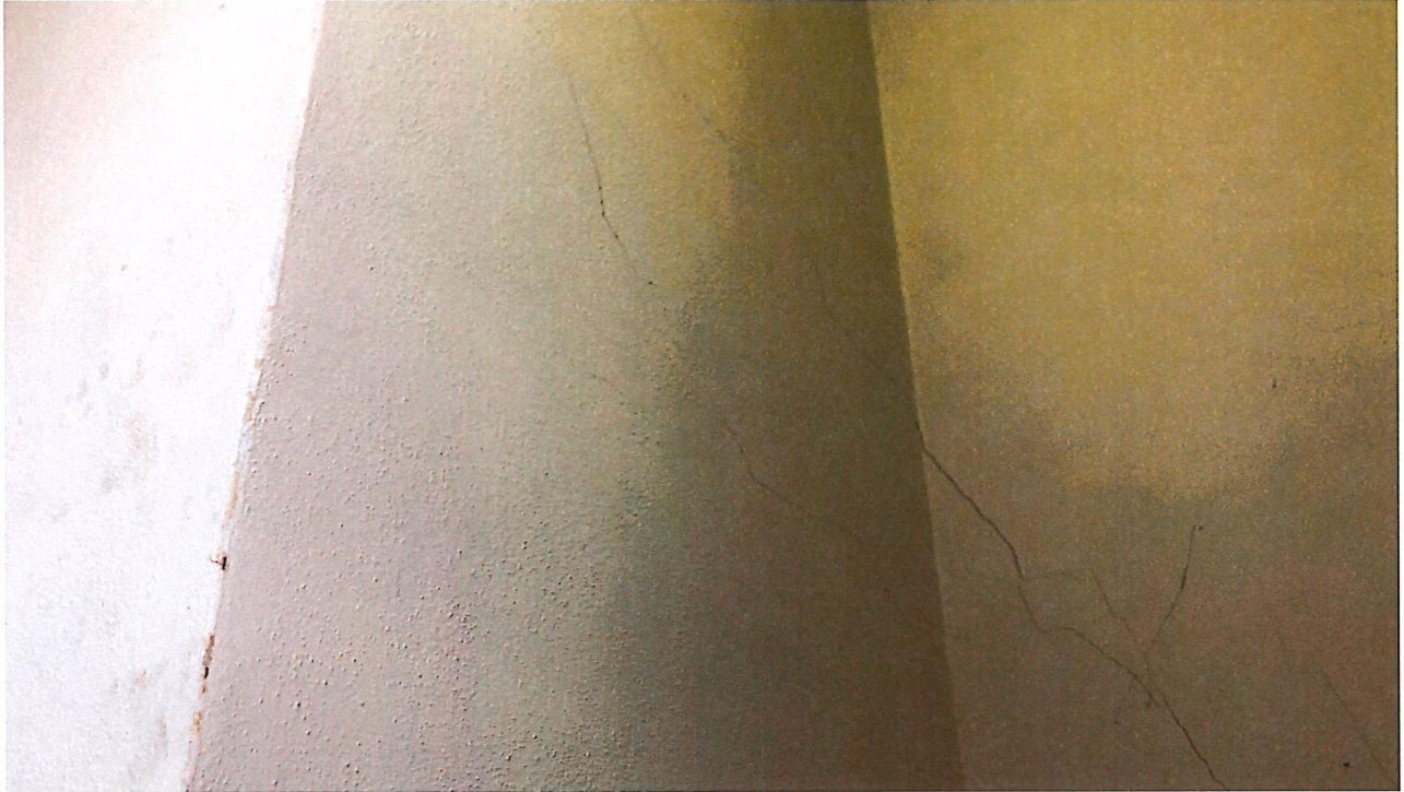
Photo 14 – Wall Crack at Stairwell of Library
