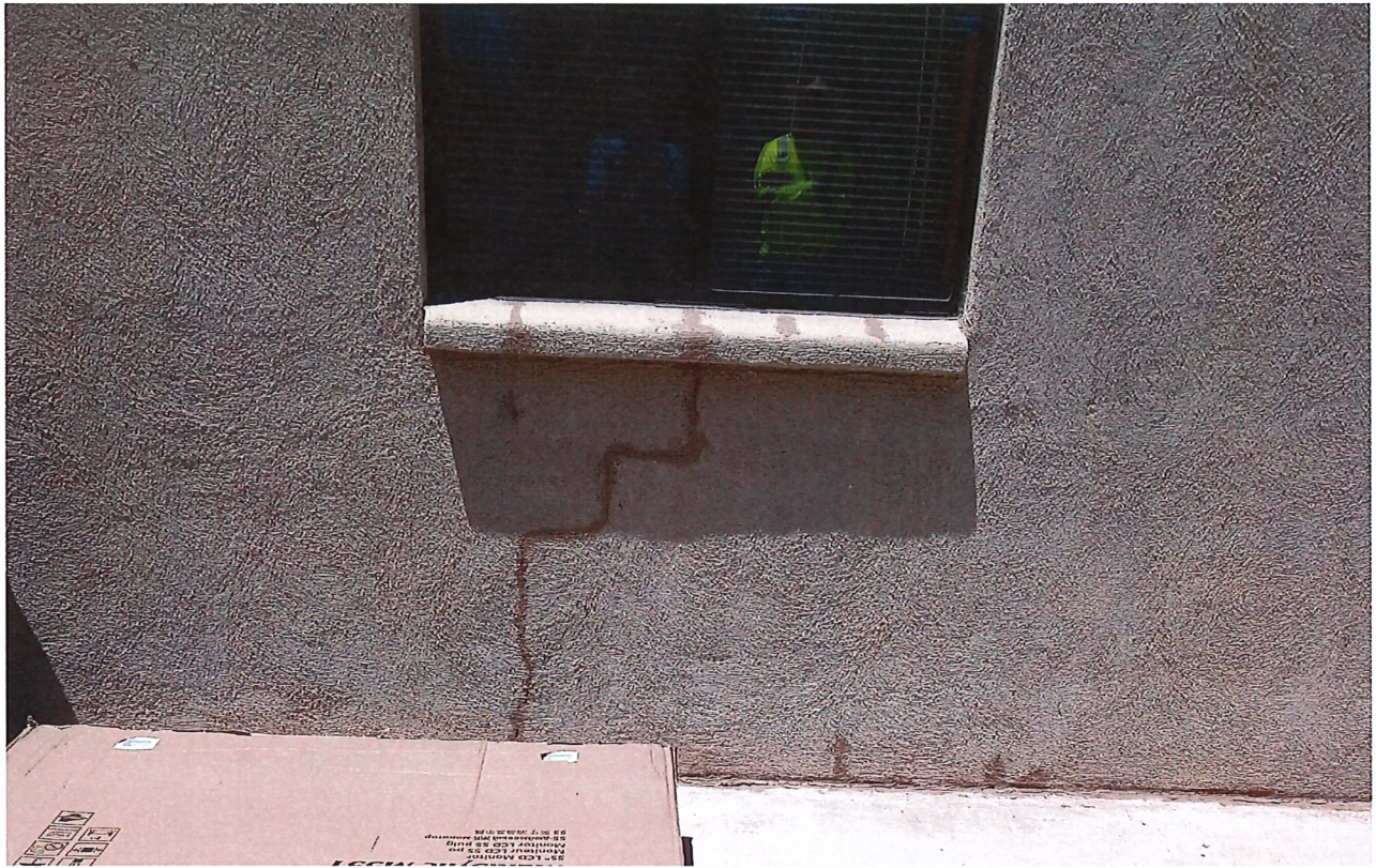
Photo 16 – Stairstep Cracks below window, Administration/Library Building
