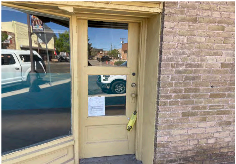
Photograph 2: Photo of LBP door and door trim.
