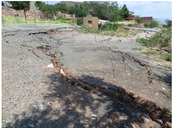
Figure 70 Photo of Jerome Landslide Related Damage
