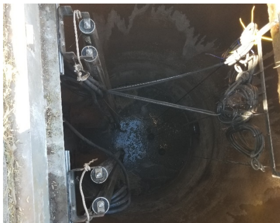
Inside of Fiesta Lift Station
