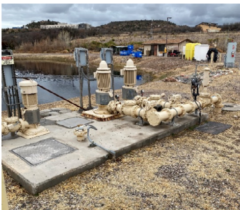
BWRf Effluent Lift Station Pumps
