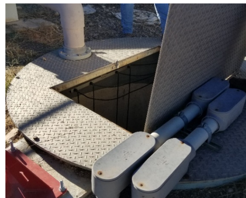
Alamos Lift Station
