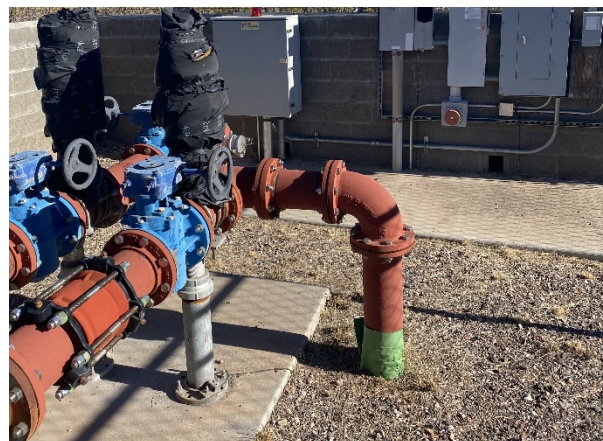
Check Valve, Gate Valve, and Air Release Assembly
