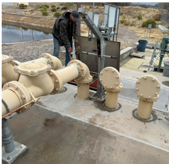
Wet Well and Discharge Piping
