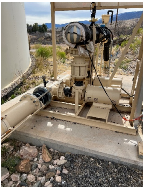
Booster Pumps and Discharge Header
