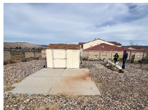
Mountain Gate Well – Treatment
