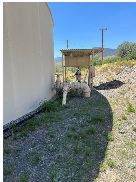
Booster Pump and Shade Structure
