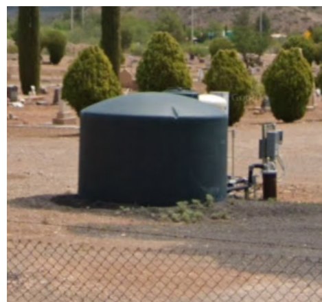
Cemetery Well Irrigation Tank
