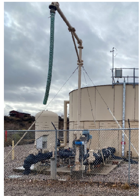
Discharge Piping and Hose
