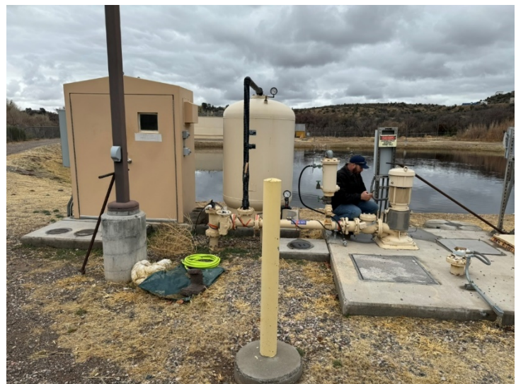
Plant Process Water System
