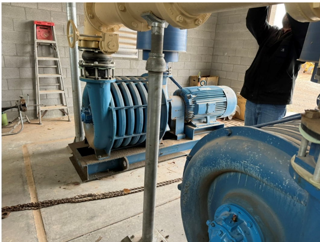
Motor and Blower
