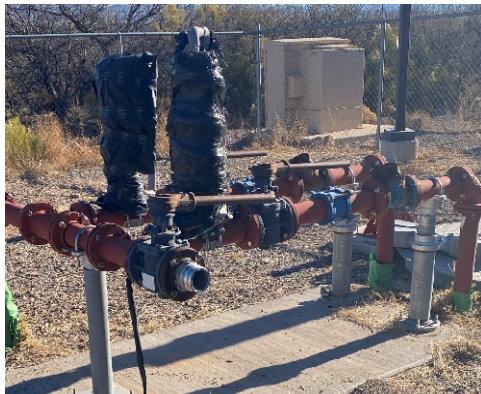
Check Valve, Gate Valve and Air Release Assembly
