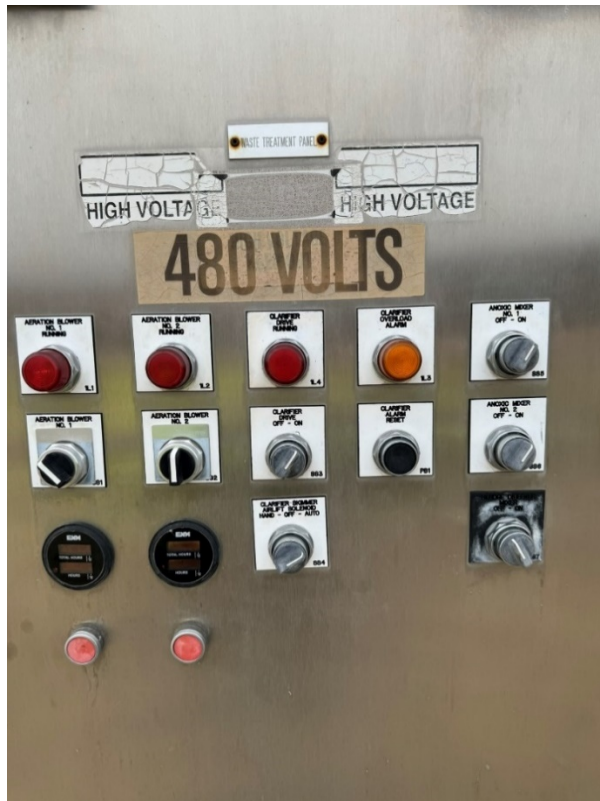
Blowers Control Panel
