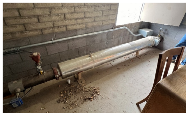
Booster Pump and Piping Assembly
