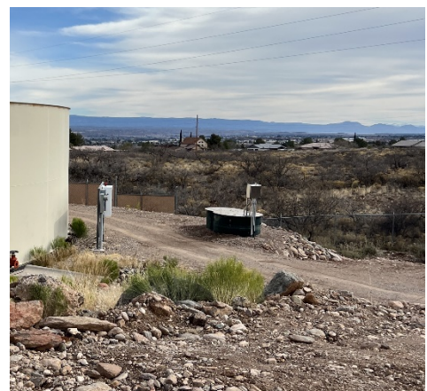
89A Lift Station Location
