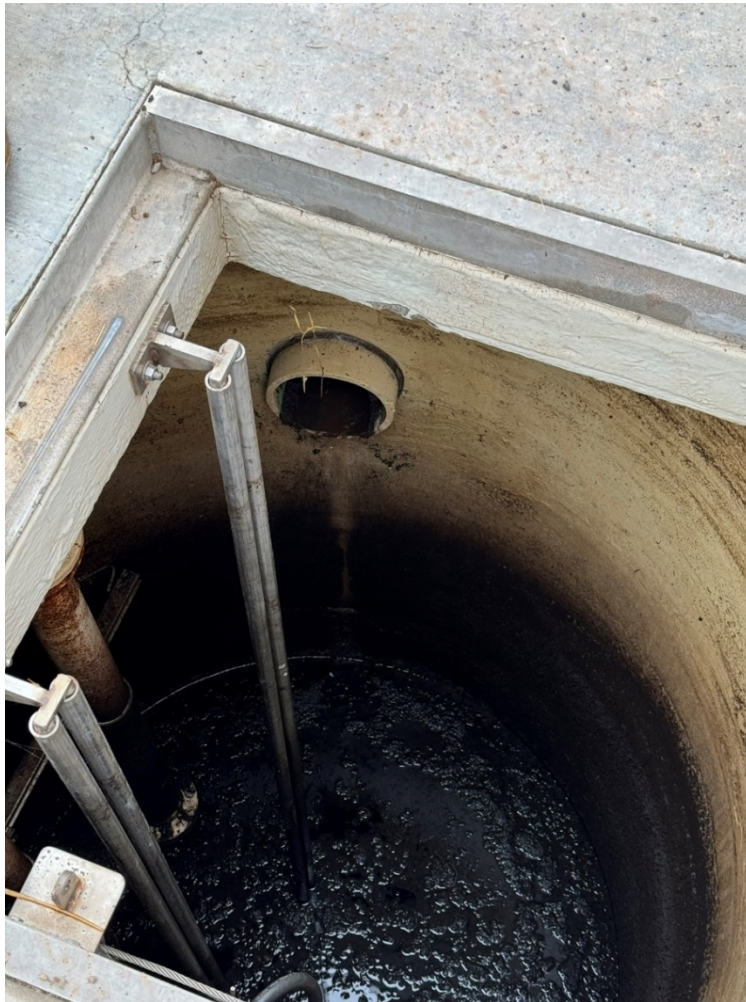
Filtrate Pump Station Wet Well Interior
