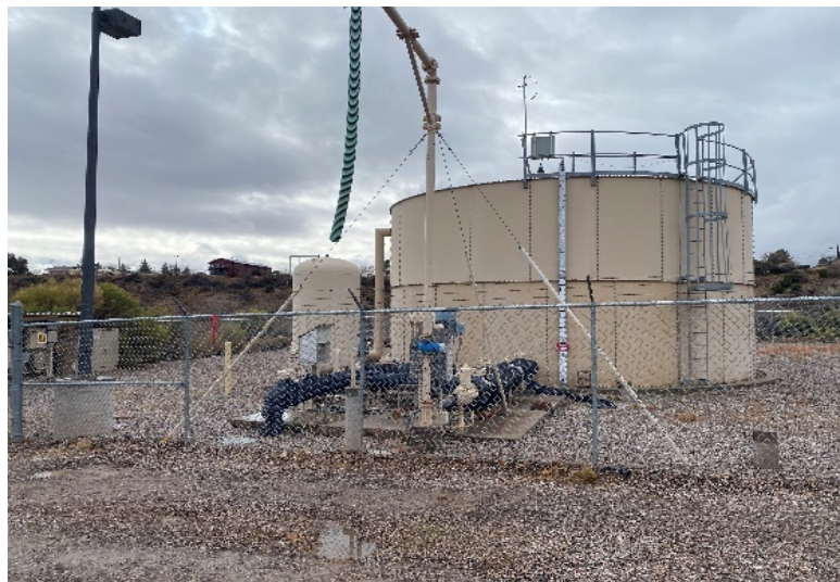
VRIC Irrigation Site Tank
