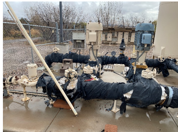
Booster Pump Station Looking East
