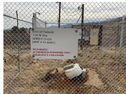
89A Well – Well Head (Inactive)
