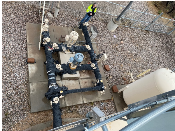
Booster Pump Station Elevated View
