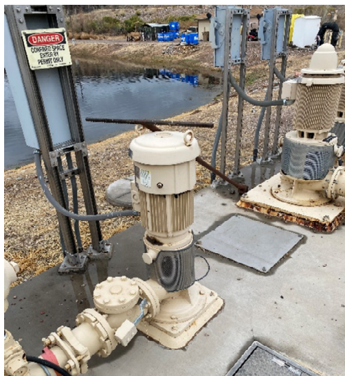
Process Water Pump
