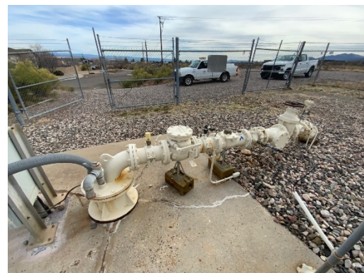
Well Head and Discharge Piping
