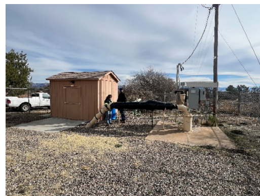
Well Head and Discharge Piping
