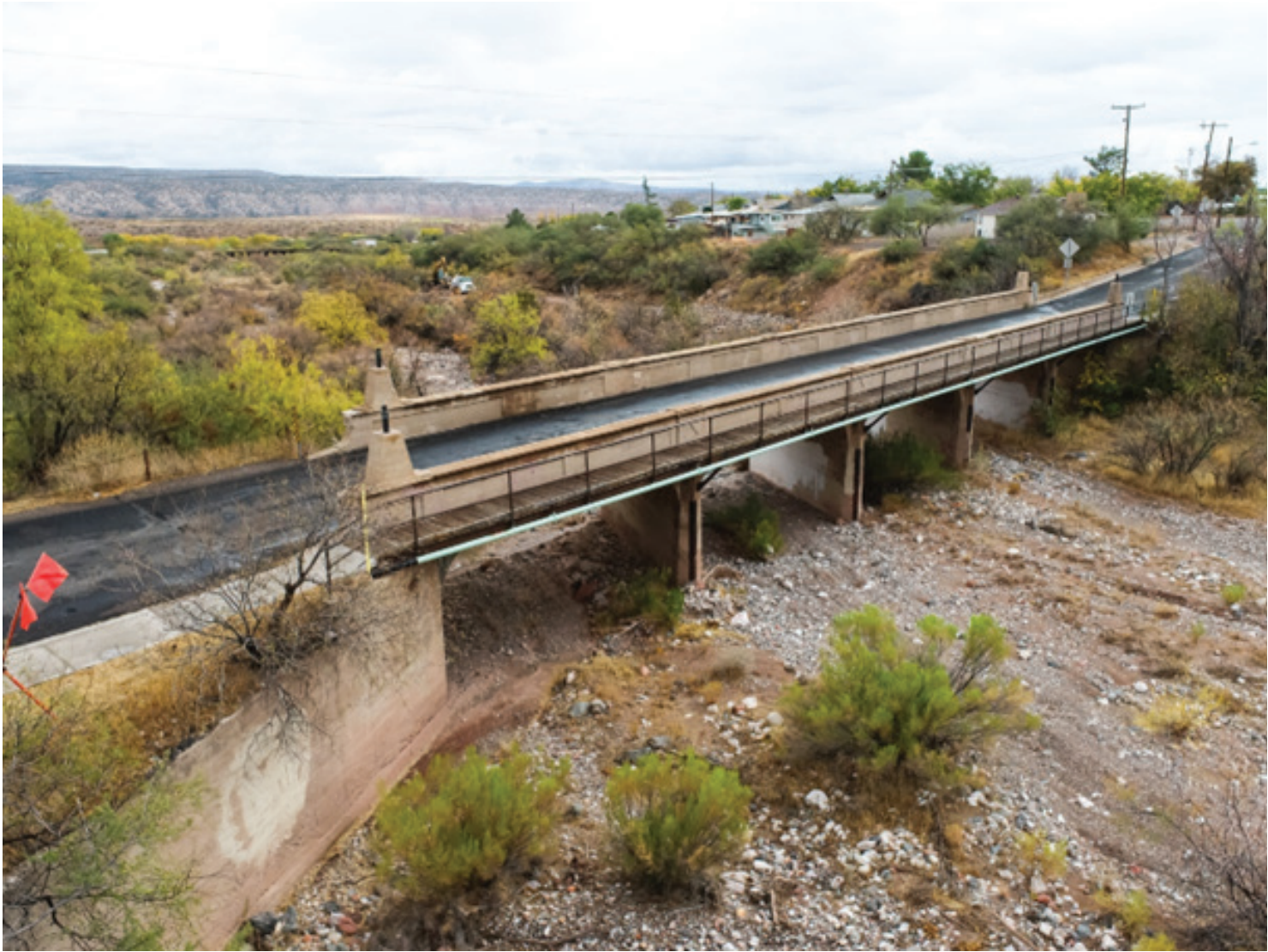
Existing Bridge Lighting
